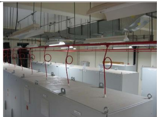
Cabinets tied together side by side using existing lifting hooks at top of cabinets
