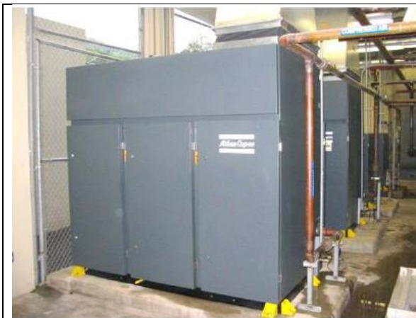
Equipment cabinets retrofitted with unidirectional snubbers at base
