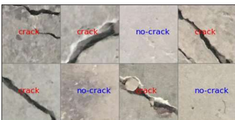
Patch level classification of cracks.
