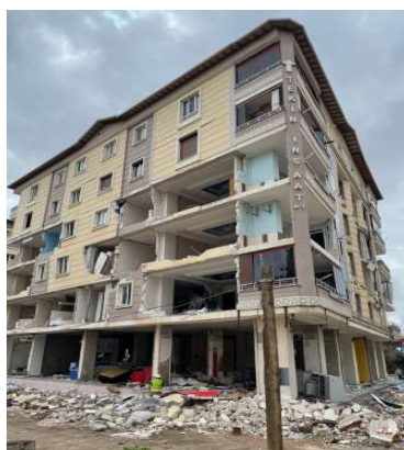
Non-structural damage in the envelopes of a residential building in Turkey (6th February 2023).
