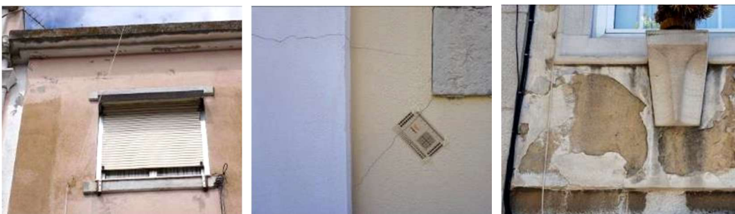
Different types of defects observed on rendered façades during visual inspections: stains, cracks and loss of cohesion and adhesion (from left to right).
