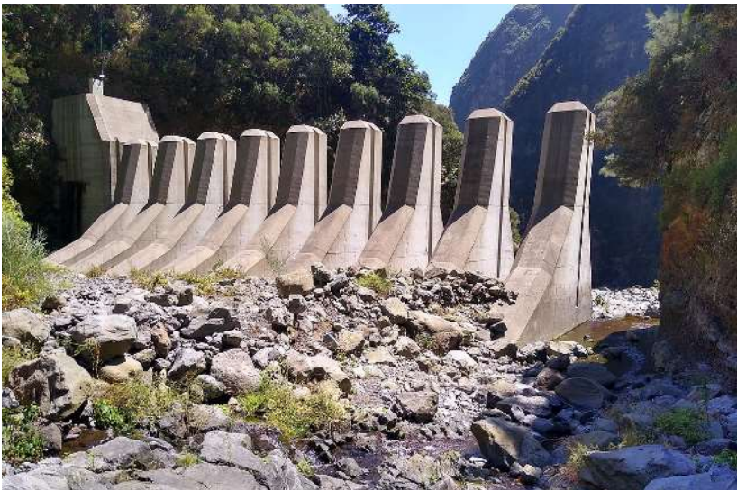
Open type check dam: concrete slit barrier of St. Luzia River in Madeira, Portugal.
