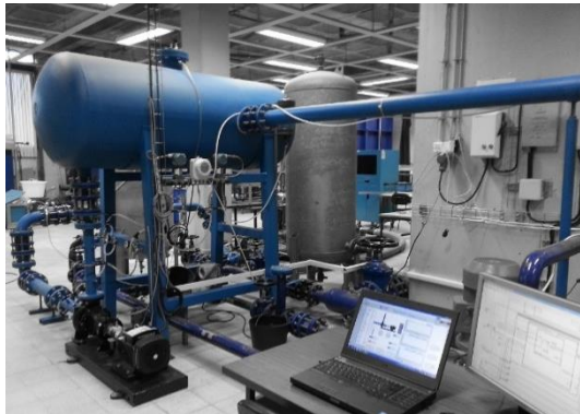
Figure 4. Test-Hydro experimental facility at IST: overall view.
