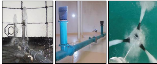
Figure 7. Inlet pipe with several flexible nozzles.
