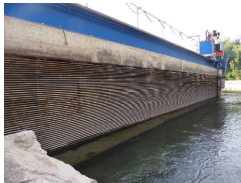
Figure 1. The horizontal bar rack bypass system at the residual flow HPP Schiffmühle, Switzerland, during revision work in July 2018.
