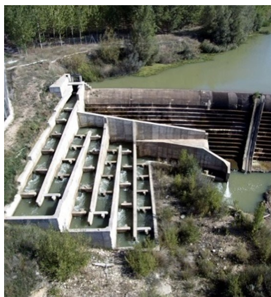
Figure 3. Aerial view of the pool-type fishway at Guma HPP.
