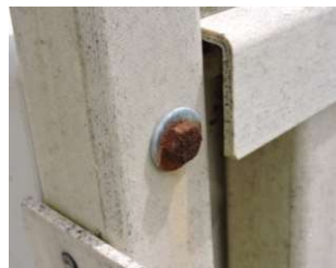
Corrosion of bolted elements
