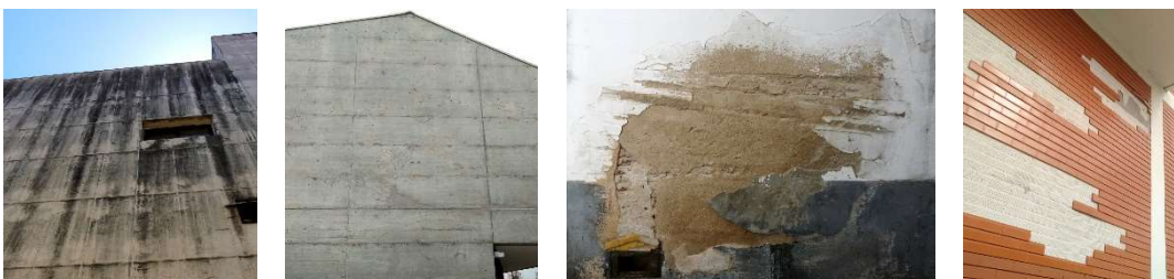
Defects in stone claddings, architectural concrete surfaces, rendered façades and adhesive ceramic tiling.
