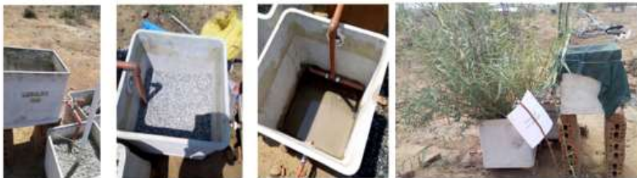
Assembly and operation of the constructed wetlands treatment system with subsequent use in crop irrigation.
