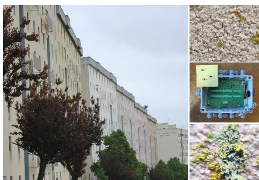
Figure 1. Evaluation of the hygrothermal conditions and of the biological colonization observed on External Thermal Insulation Composite Systems (ETICS).
