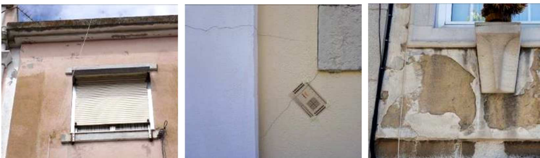
Different types of defects observed on rendered façades during visual inspections: stains, cracks and loss of cohesion and adhesion (from left to right).
