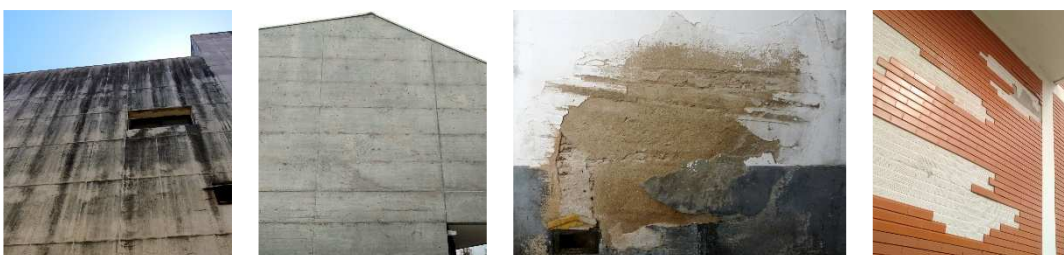
Defects in stone claddings, architectural concrete surfaces, rendered façades and adhesive ceramic tiling.
